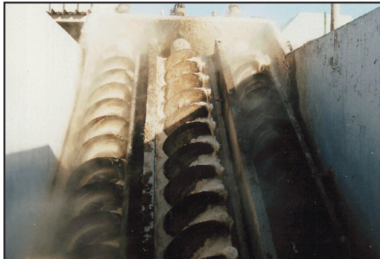
Three effluent pumps in operation prior to repair
